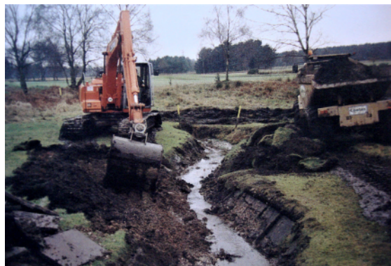
Drainage system to take water to the river Leen.
